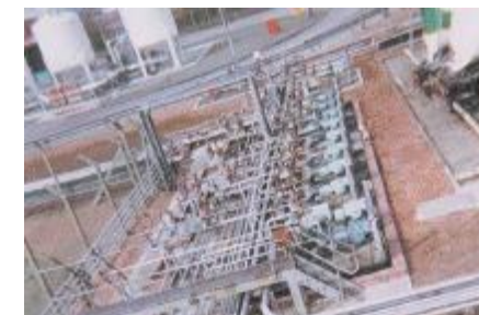
BP Oil Grangemouth, Scotland Tanker Terminal, additive injection pump platform and vapour recovery unit.
