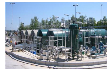
Farnborough Airport New Aviation Tank Farm
