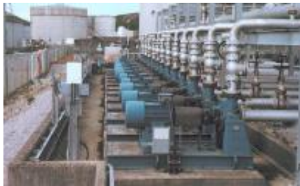
Pumping system design and installation
