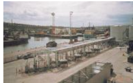
BP/Shell J.V. Aberdeen Terminal redevelopment showing truck bottom loading facilities
