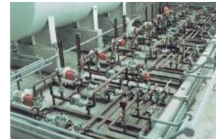
Multi-user additive pressuring pump skid units design and installation
