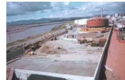
Ross Chemical Storage Co, Grangemouth demolition and construction of 3 new storage tanks and impervious bund
